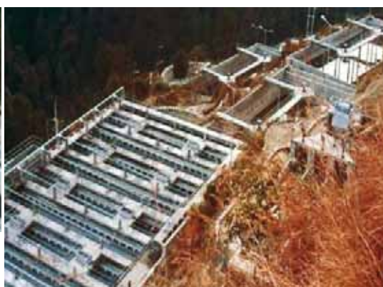
Sewage Treatment Plant at Summerhill, Shimla
