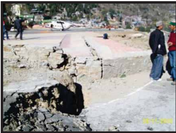
Reckong Peo Landslide
