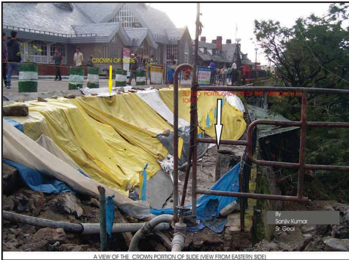
A VIEW OF THE CROWN PORTION OF SLIDE (VIEW FROM EASTERN SIDE)
