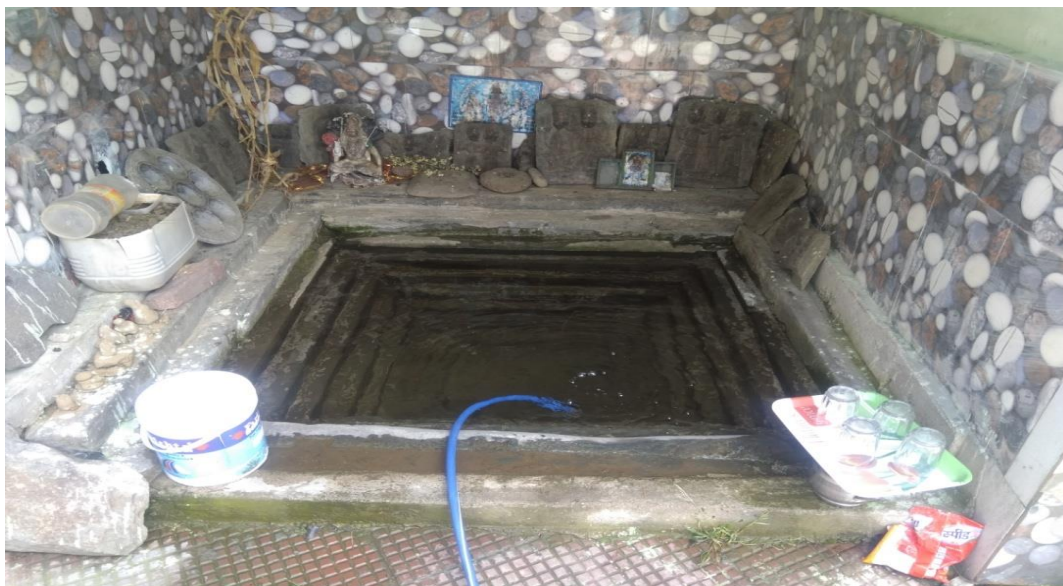
FIGURE 16 DRIED SPRING USED AS STORAGE TANK
