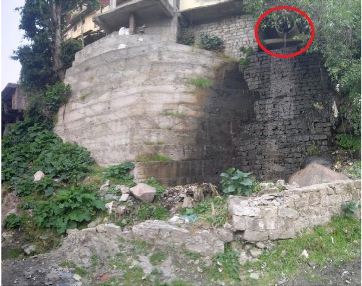
FIGURE 23 SEWAGE PIPELINE DIRECTLY DRAINS INTO RIVER STREAM
