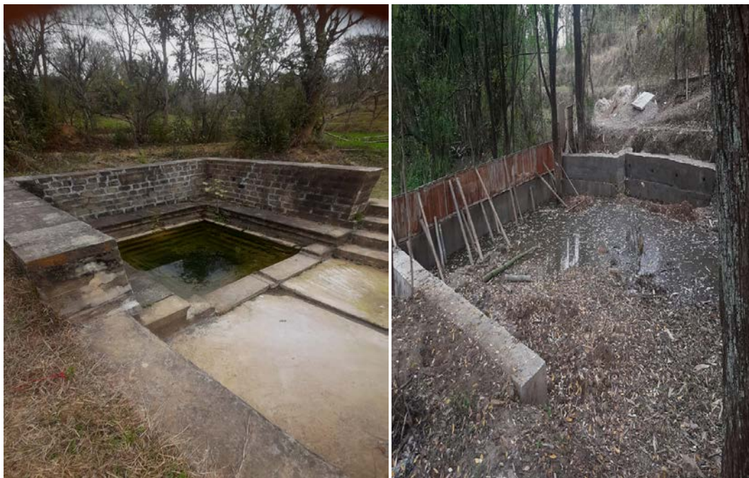
Figure 9 Construction of new bawari in village Lag, GP Manvi, Block Bhoranj, Hamirpur.
