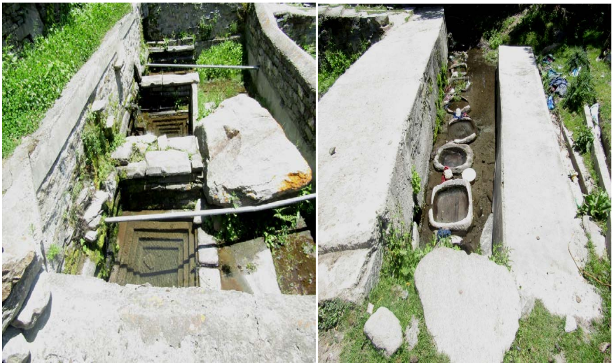
Figure 8 Construction, maintenance and protection of natural water source in village Kamru, Kinnaur.
